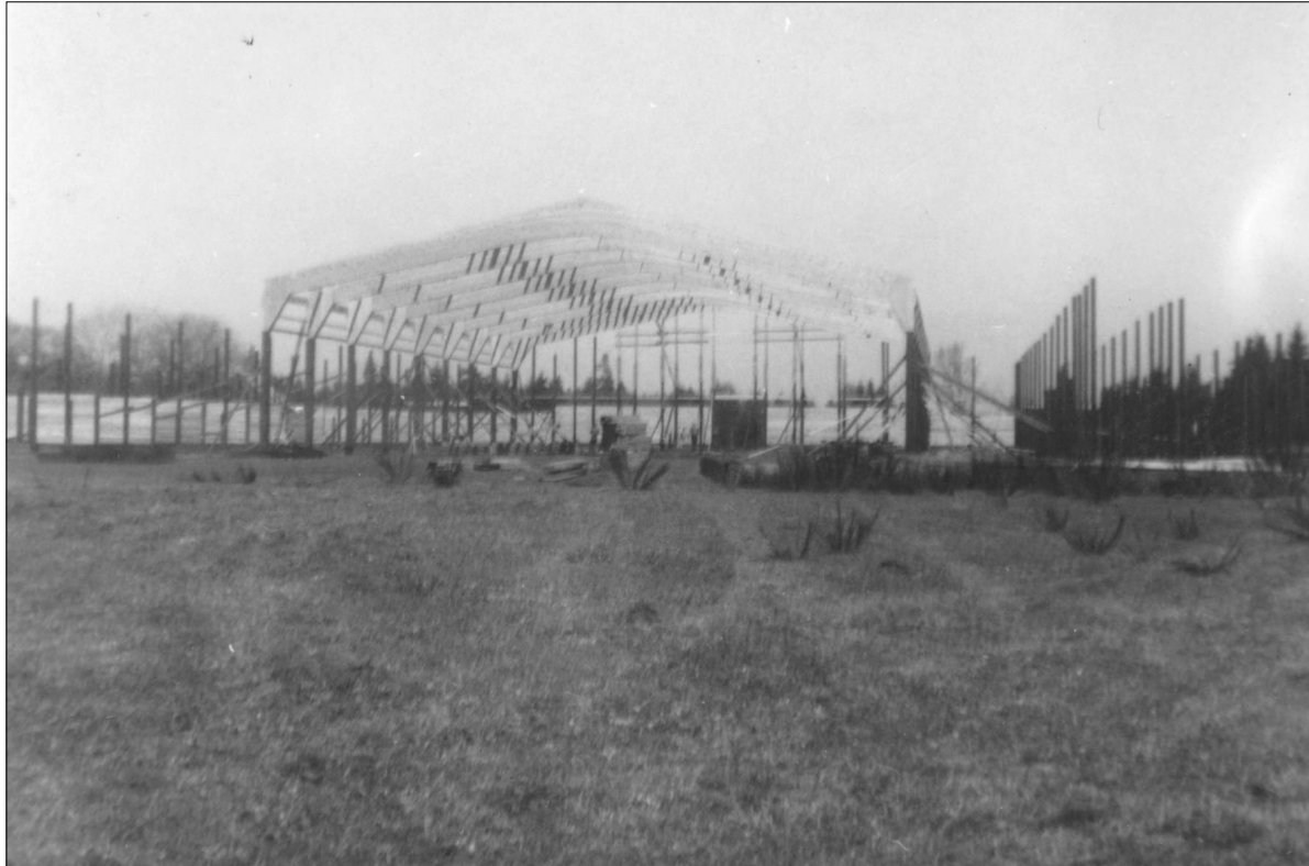
The large arena at Trails End Stables as it was being built in 1965. The building contained a 200' by 90' clear span arena with seating for about 2,000. With stalls, lobby, and waiting areas, the building measured 256' by 190' overall.
